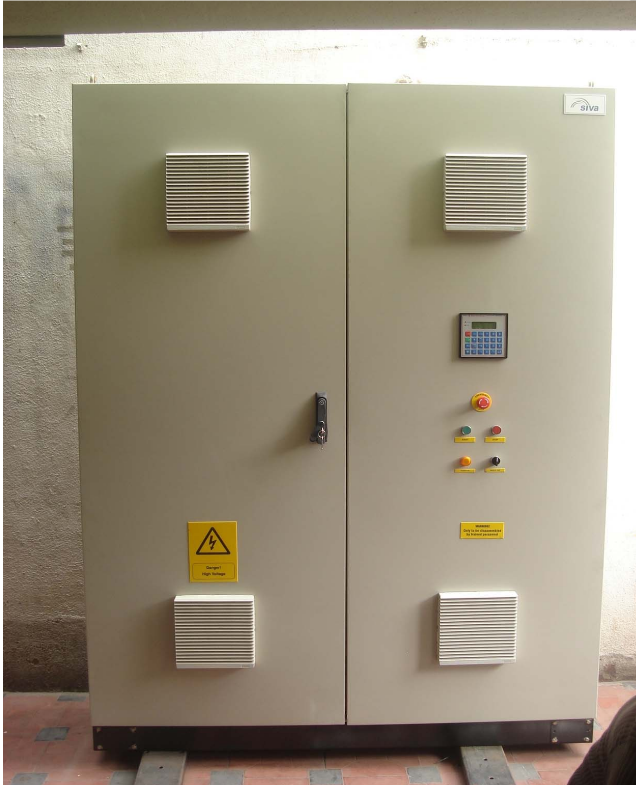
FRONT VIEW OF 250/50 KW CONTROL PANEL
