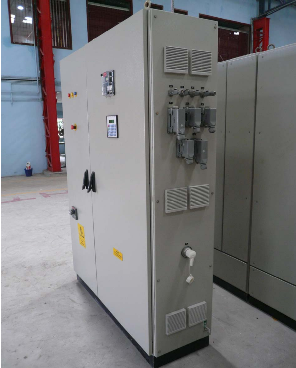
SIDE VIEW OF 250/80KW CONTROL PANEL
