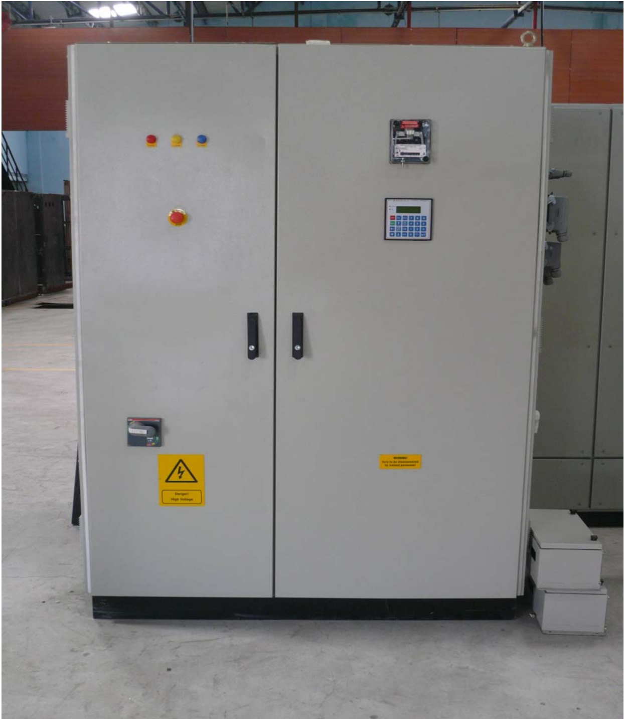
FRONT VIEW OF 250/80KW CONTROL PANEL WITH TOP BOXES 1& 2
